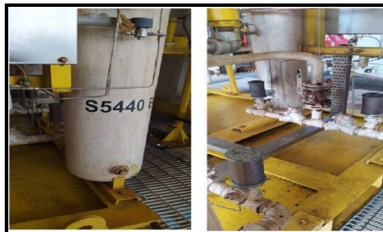
Air leakage on the existing silencer / muffler
