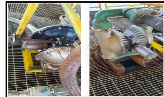
High noise emitted from pump due to poor NEC maintenance
