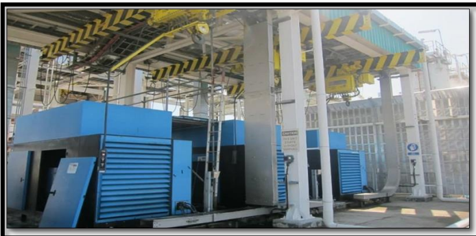
Damage door (acoustic enclosure)
