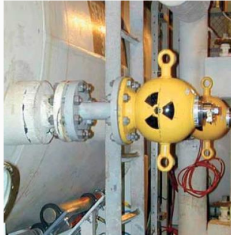
Radiometric gauges (density, level etc) with sealed source
